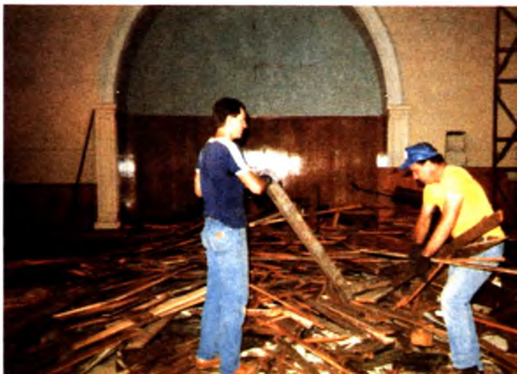
Tim Tarkas and Wayne Lynch begin removing partitions and other rubble from the century-old structure in June 1987.
